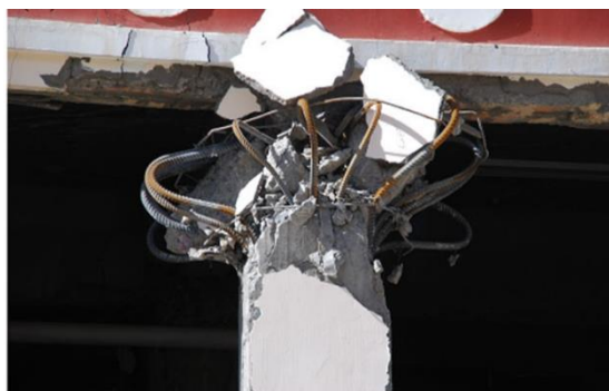
(b) Yushu earthquake of 14th April 2010, China Qinghai (Gong et al., 2015)
