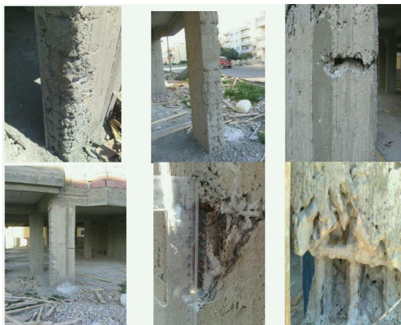
Figure 1: Honeycombing and insufficient vibration problems in columns
